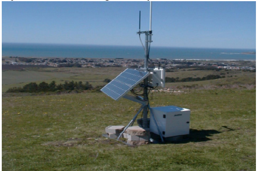
Example Solar Powered MetroMesh Router Installation
